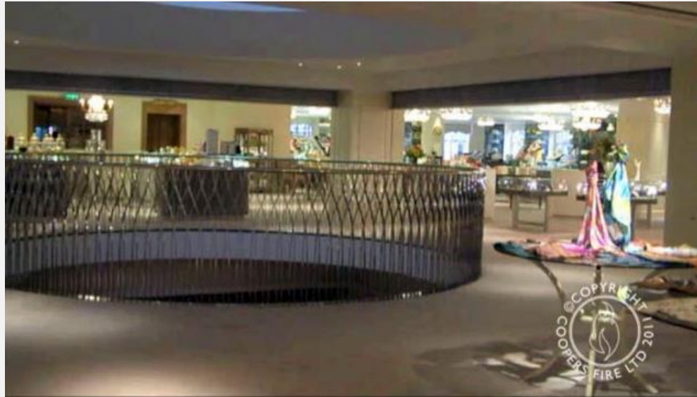
Atrium - FireMaster Fire Curtains, Fortnum & Mason, London
