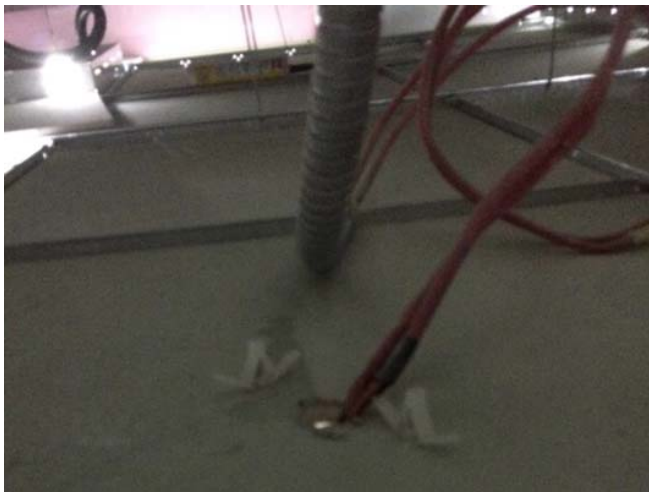
Smoke detector without back box
