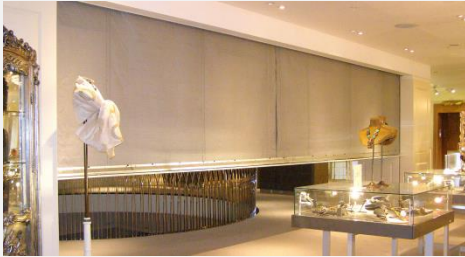
Vertical Fire Curtain
