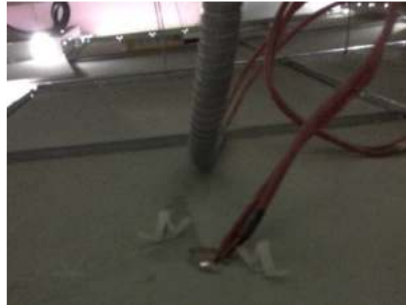
Smoke detector without backbox
