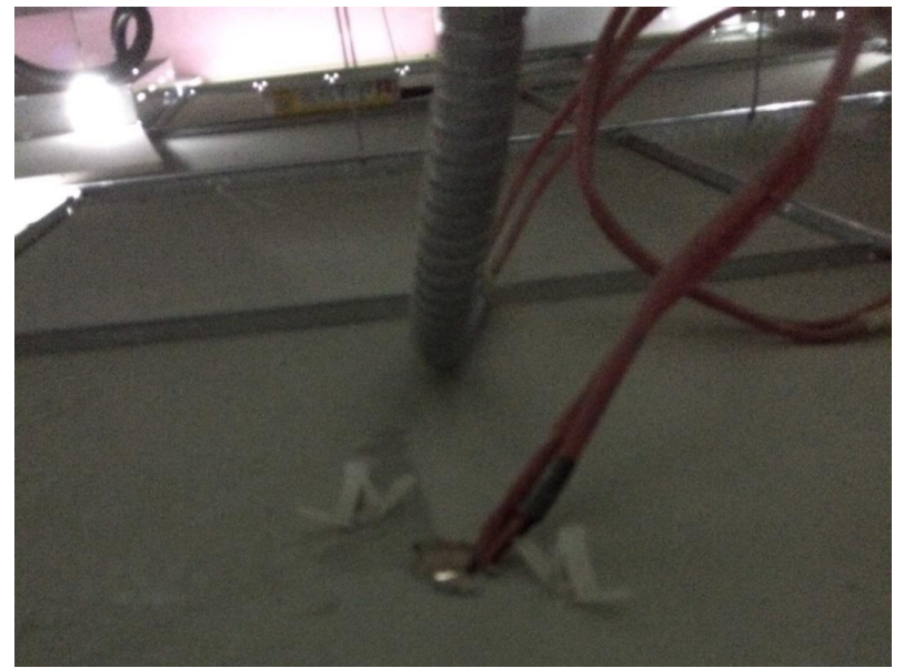
Smoke detector without backbox
