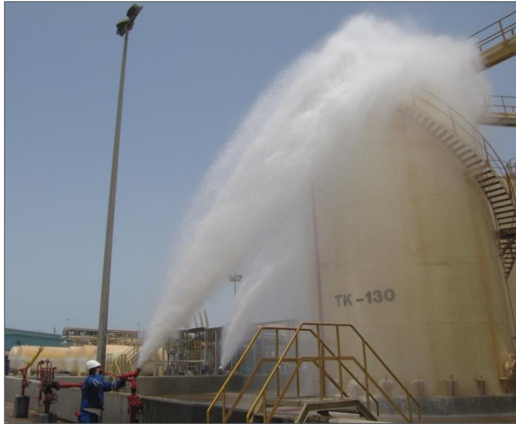
Fire Main Flow Testing
