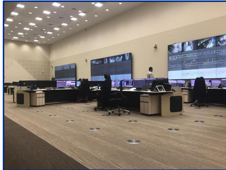
Integrated Control Centre – BACS to SCADA
