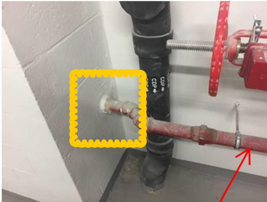
Sprinkler Alarm Check Valve Drain Pipe.
